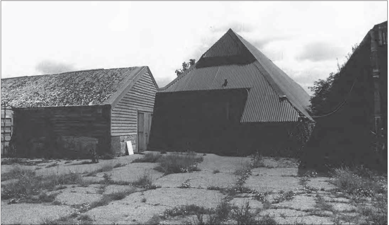
Appendix 4.12: Exterior view of the southern barn from the west, taken in 2000 (image cropped top/bottom). © English Heritage NMR Ref.: AA030280.
